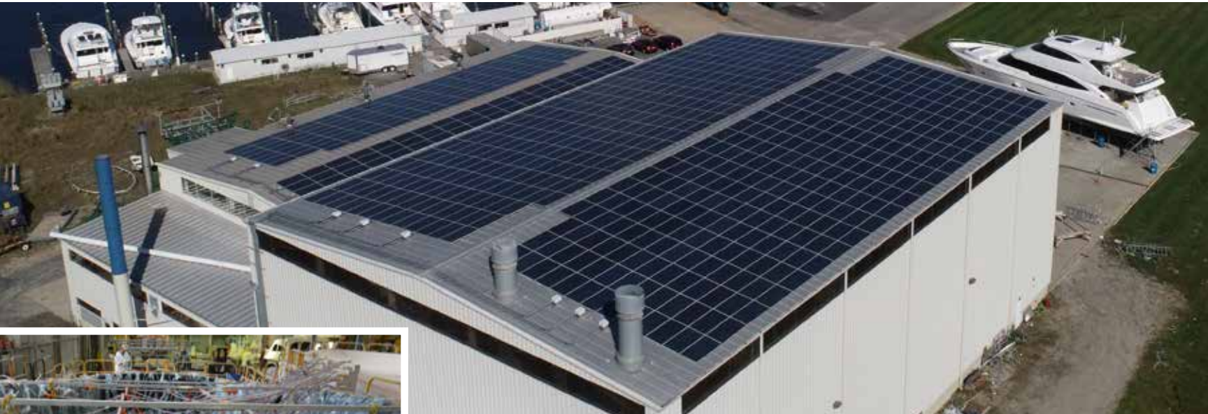
An aerial view of Building 5 and 5A's solar panels.
